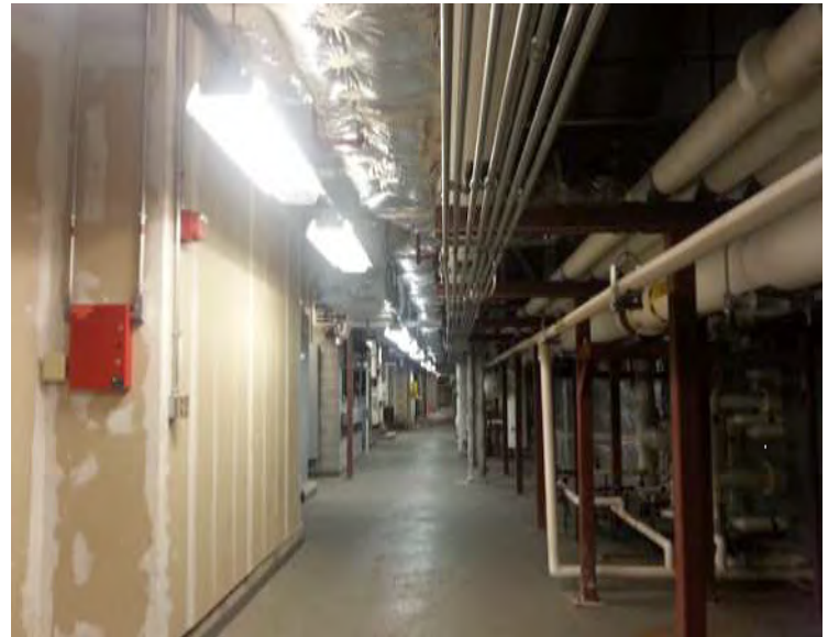
Figure 7. During the Annex Re-tuning building walk-through, operators found lighting in this mechanical room always on
