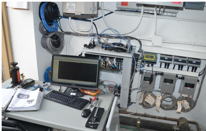
Figure 7 – Setup at Tampa site during testing of installation
