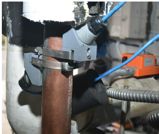
Figure 3 – Installed ultrasonic water flow meter in Z-formation
