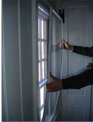
Figure 2 | Interior storm windows installed to support original windows (photo courtesy of: Environmental Window Solutions, LLC.)
