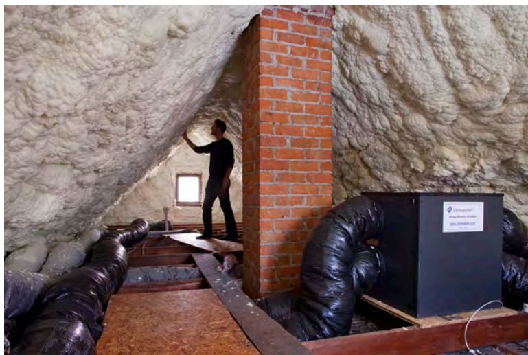
Figure 3| Spray foam insulation as approved, after successful appeal by homeowner, by Michigan SHPO (photo courtesy of: Matt Grocoff)
