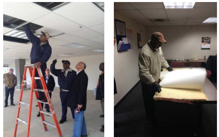
Figure 4. Building walk-down included checking above the ceiling for duct condition, etc. (left) and reviewing electrical and mechanical prints (right)
